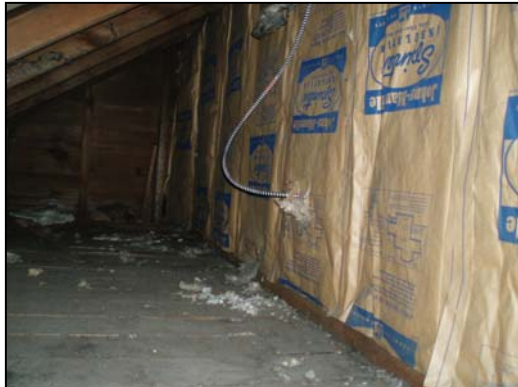
Rock Wool insulation in attic kneewall is in good shape and was installed very well. This product was produced late 50's and early 60's and most likely installed around that time. I contacted the manufacturer and there is no asbestos in this insulation.
